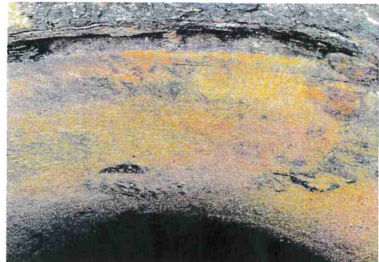
INTERNAL WALLS OF FIBERGLASS HOLDING TANK
