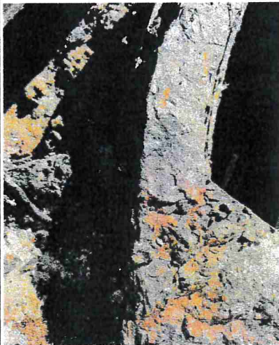
STEEL CHECKER PLATE COVER OF FIBERGLASS TANK
