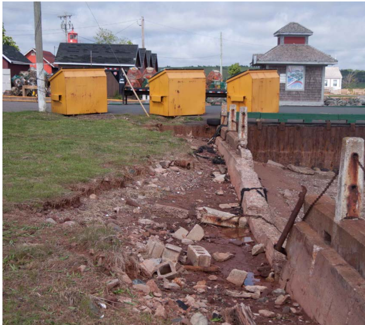
Figure 16 - An eroded segment of sea wall below 27 Water Street allows free passage for storm surge to flood the area (photo credit: D. Jardine).
