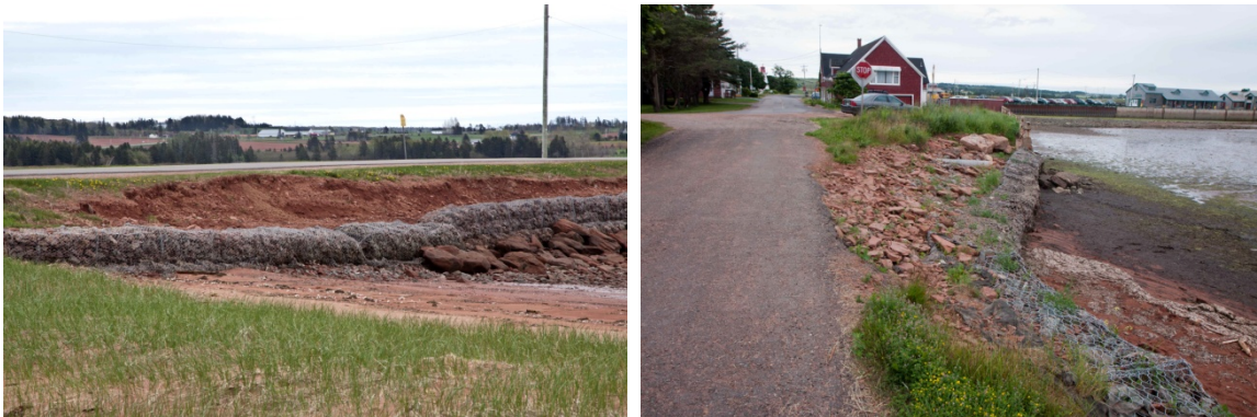
Figure 13 - Shoreline protection (gabion baskets) installed below the Causeway Road, west of Victoria Bridge (left) and at the western extent of Water Street (right) (photo credit: D. Jardine).
