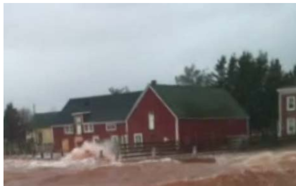
Figure 14 - Storm surge at 25 and 27 Water Street easily breached the degraded sea wall during a storm on Dec 6, 2010 (photo credits: P. Nishimura and K. Boulter).
