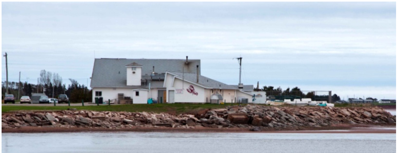
Figure 20 - Shoreline protection (rip rap composed of discarded concrete) borders the shore below Morning Star Fisheries Ltd, east of Victoria Bridge (photo credit: D. Jardine).
