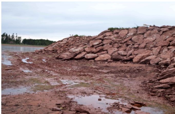
Figure 21 - Shoreline protection (sandstone) installed at Dunrovin Shores subdivision, west of the Victoria harbour front (photo credit: D. Jardine).
