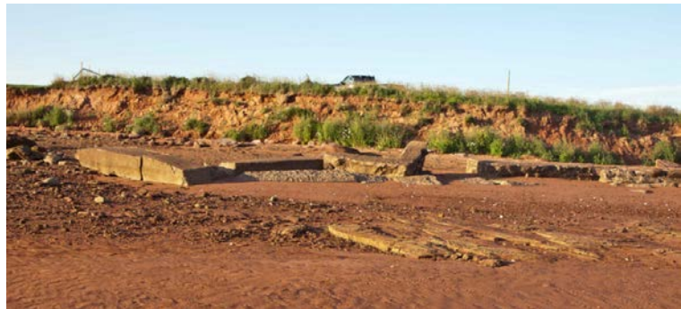
Figure 2 - Foundation of former MacDonald house now on the beach (photo credit: D. Jardine).
